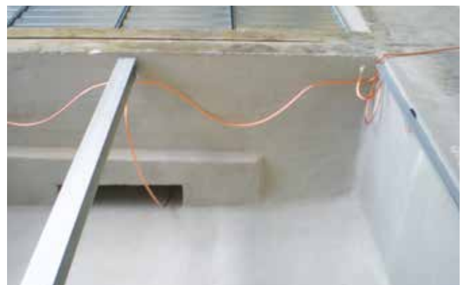
Protective grounding of the components
